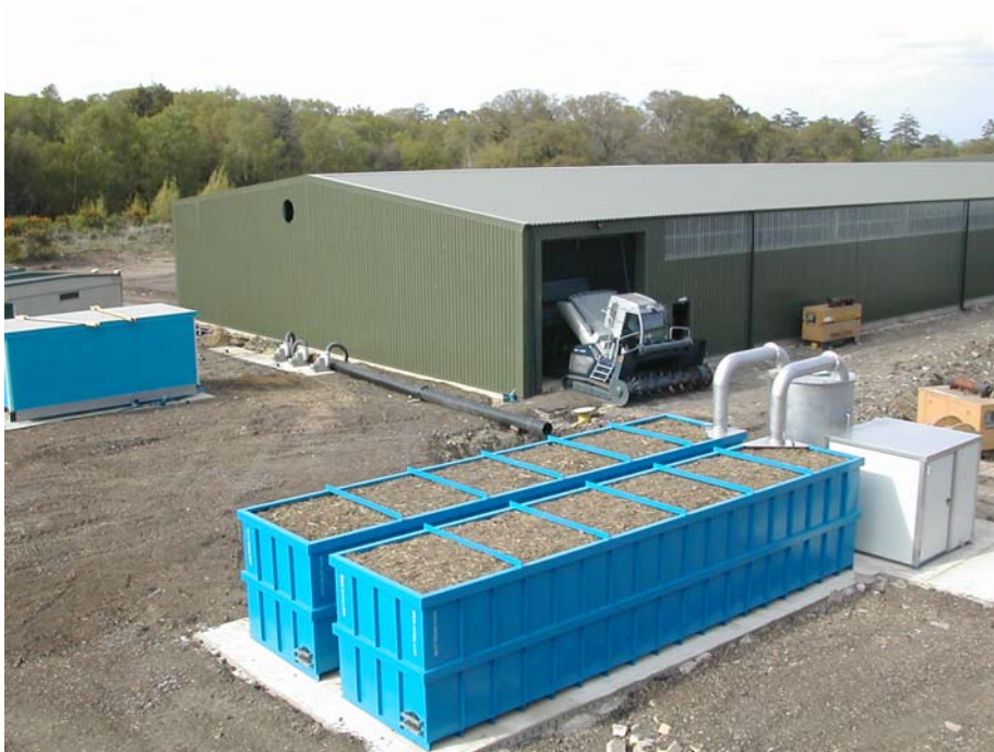
Plate 1 New Earth Technology showing biofilter and scrubber in foreground and composting hall in the background with the windrow turner emerging from the hall.
